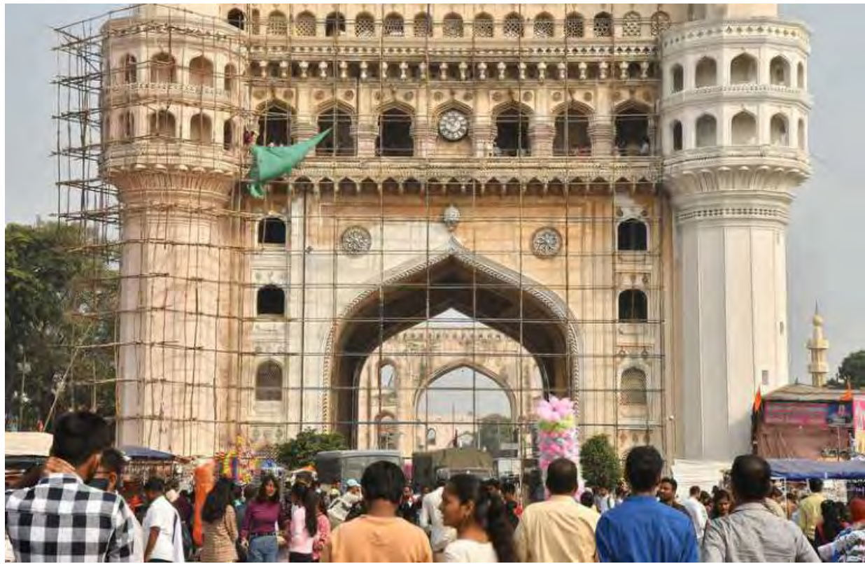
Under repair: The Archaeological Survey of India has taken up the restoration of the 432-year-old Charminar in the old city of Hyderabad on Monday. Tourists are unable to get a full-size view of the monument at present. NAGARA GOPAL
