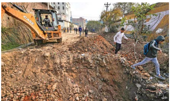
Commuters walk past a road dug up to prevent the movement of heavy vehicles in view of the farmers' march near the Singhu border in New Delhi on Wednesday. — PTI
