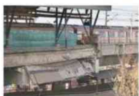
At Gokulpuri Metro station after the wall collapse on Thursday. Tashi Tobgyal RELATED REPORTS PAGE 3
