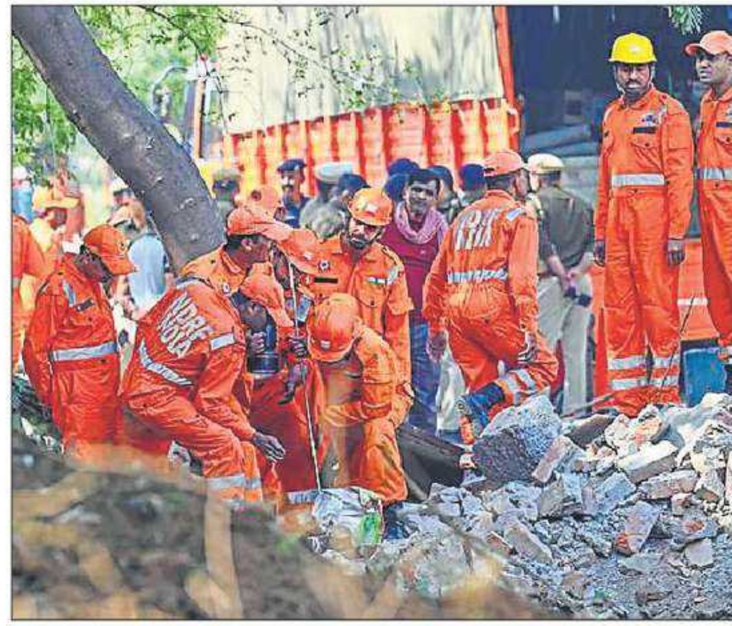
NDRF personnel take part in the rescue operation at DJB's sewage treatment plant in Keshopur on Sunday. SANCHIT KHANNA/HT
