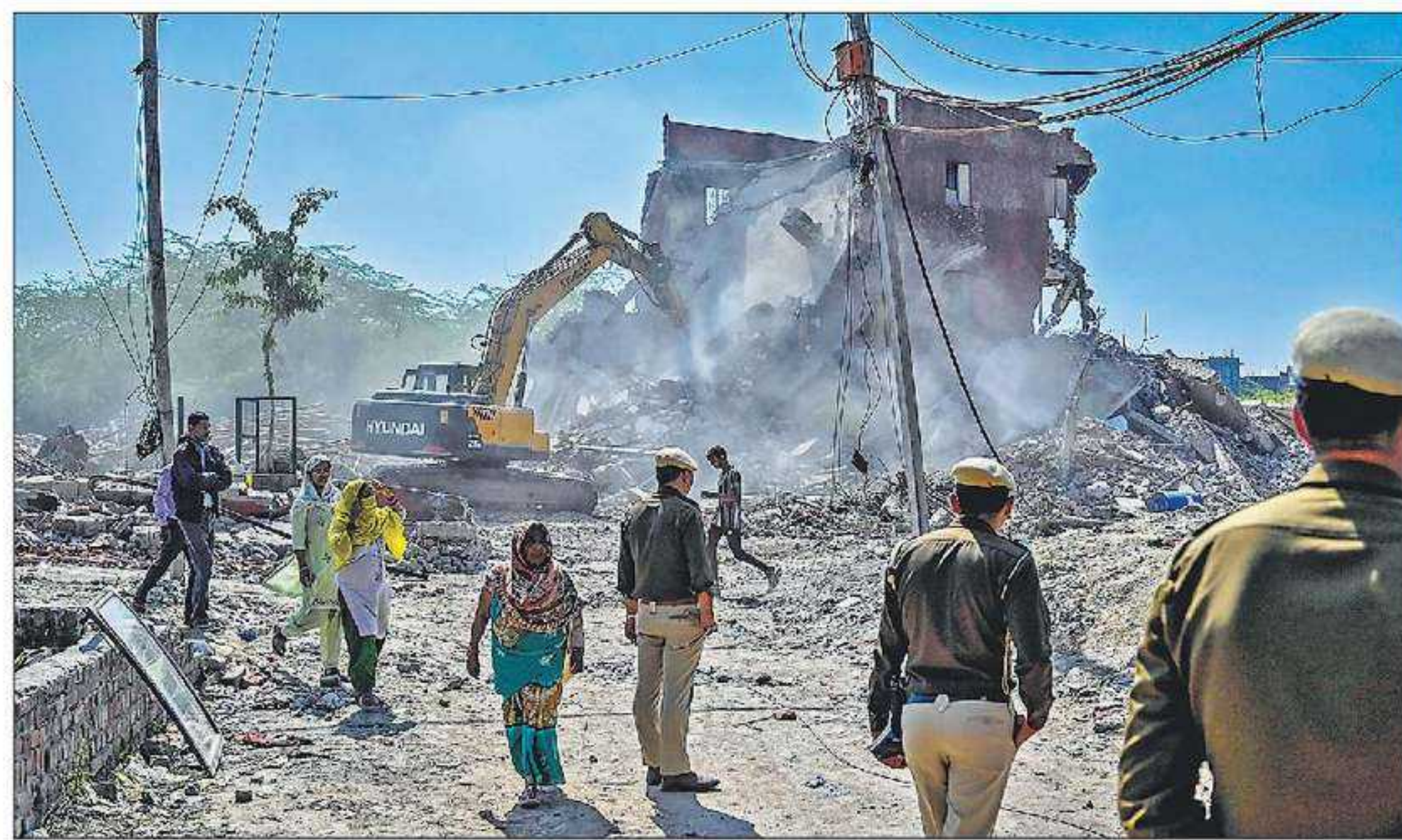
The forest department continued its demolition drive in the Southern Ridge on Thursday, freeing up one acre of forest land in Sangam Vihar and Chhatarpur. Forest officials said they have removed encroachments from 8 acres of forest land in south Delhi over the last five days. RAJ KRAJ/HT
