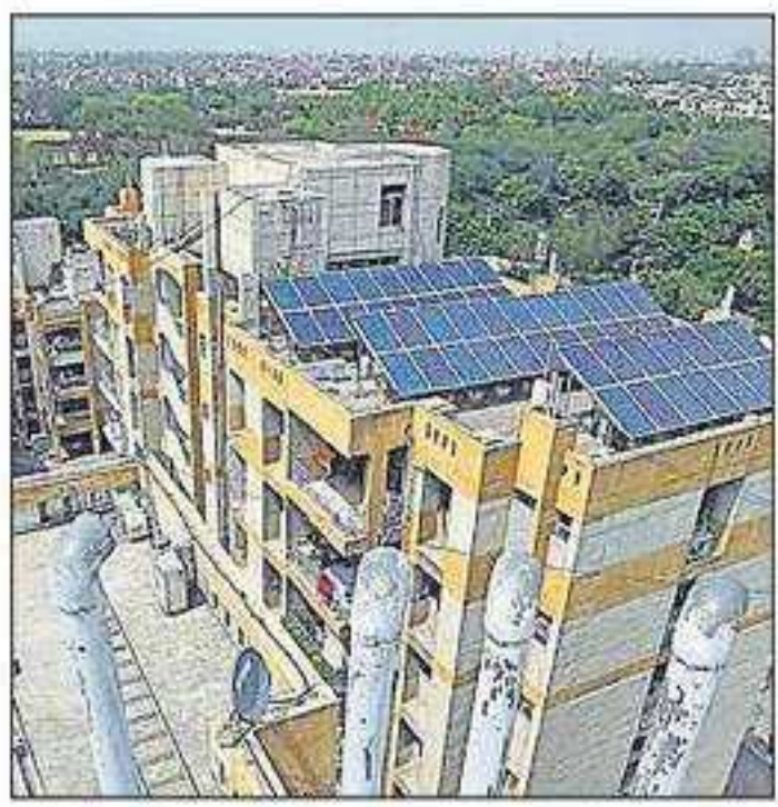
These installations will result in an additional 30 GW of solar capacity.
