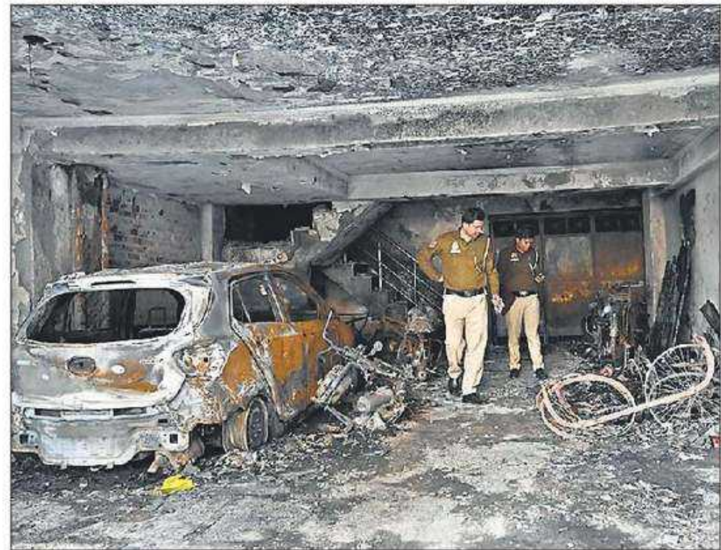
Charred vehicles in the stilt parking of the building.
