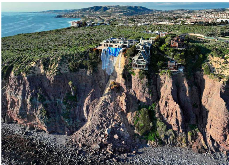
An aerial view of mansions still standing along a cliff after a portion of the cliffside tumbled into the Pacific Ocean following days of heavy rains on February 27, at Dana Point, California. A powerful atmospheric river brought flooding, mudslides, and over 17 cm of rain - half the average yearly total. Such atmospheric rivers have been destroying the coveted coastal cliffs. AFP
