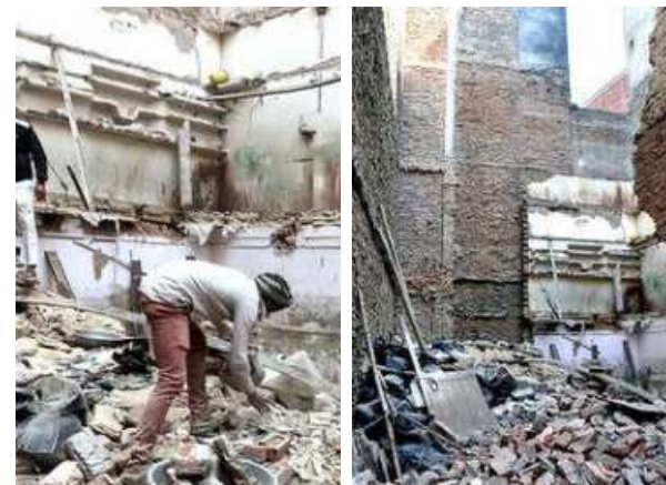
Picking up the pieces: The three employees were working at the factory housed on the ground floor of the building. SUSHIL KUMAR VERMA
