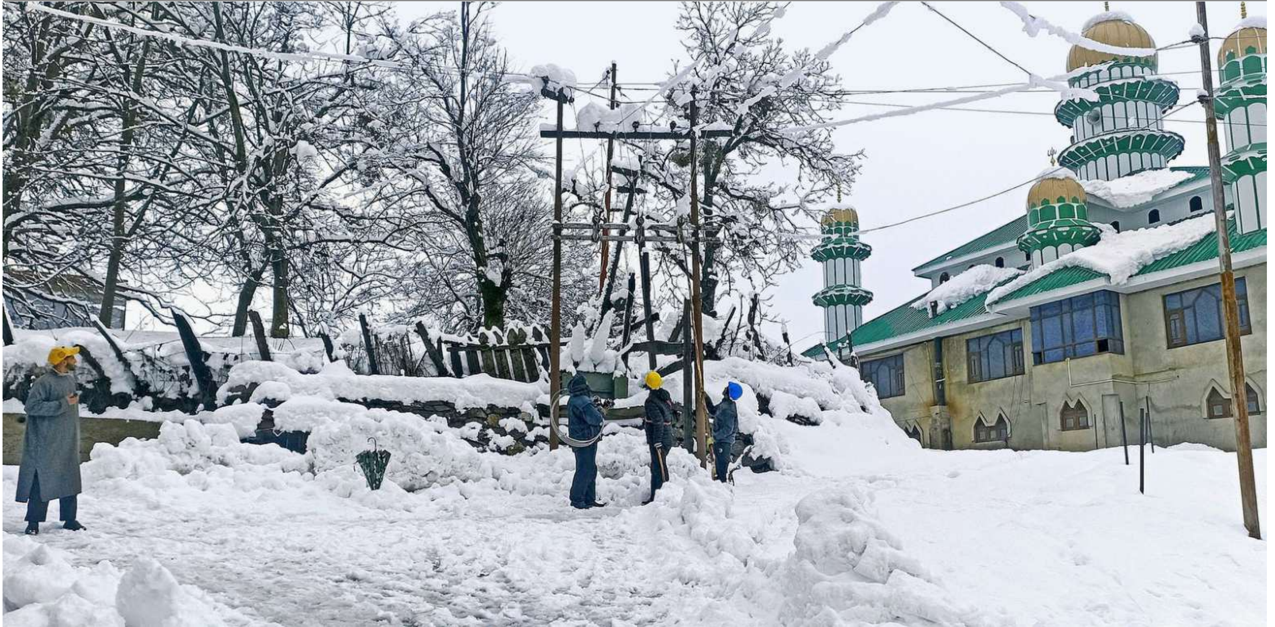
Lights out: Employees of the Power Development Department repairing an electric line during heavy snowfall at Kukroosa in Kupwara district in February this year. J&K's power generation capacity is around 3,633 MW, far below its potential of 18,392 MW. FILE PHOTO
