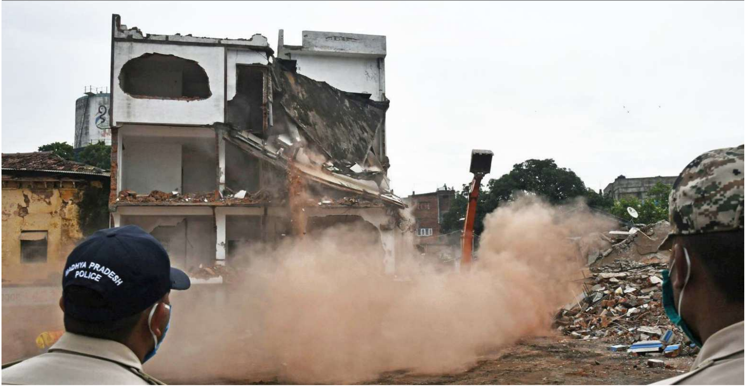
Swift action: A building belonging to Pyare Miyan, a 68-year-old man accused of raping minor girls and running a sex racket, being demolished by the district administration in Bhopal on July 14, 2020. He was convicted in the case and sentenced to life imprisonment in 2022. A.M. FARUQUI
