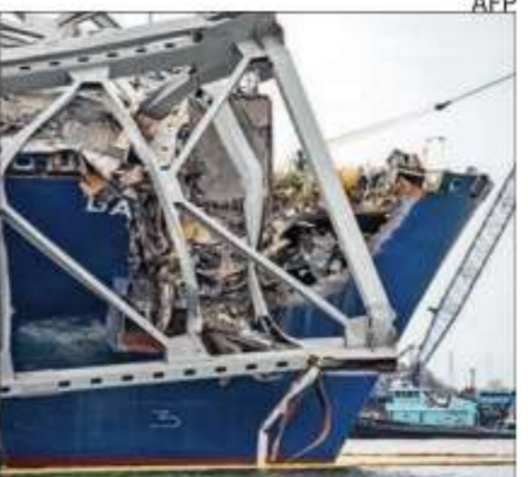
A portion of the collapsed Francis Scott Key Bridge
