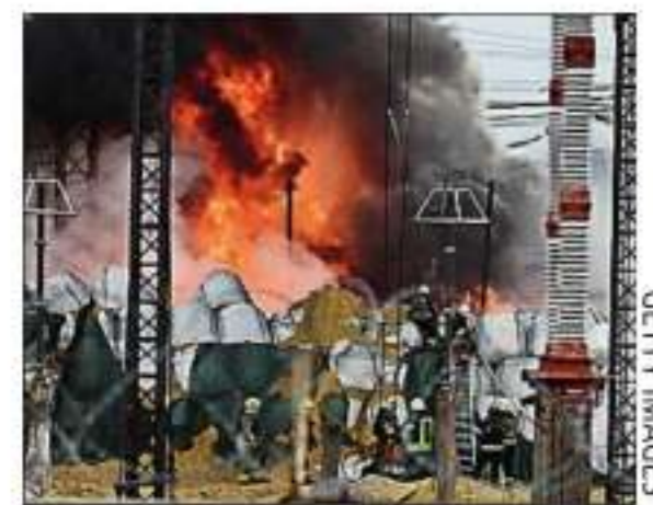
Firefighters extinguish a blaze at an electrical substation after a massive strike in Kharkiv
