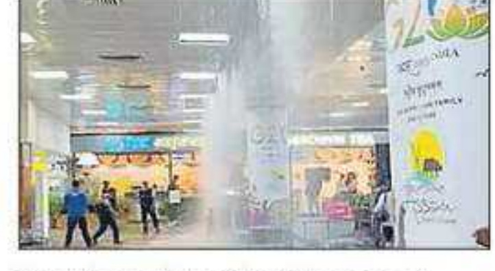
Portion of roof collapses at Guwahati airport.
