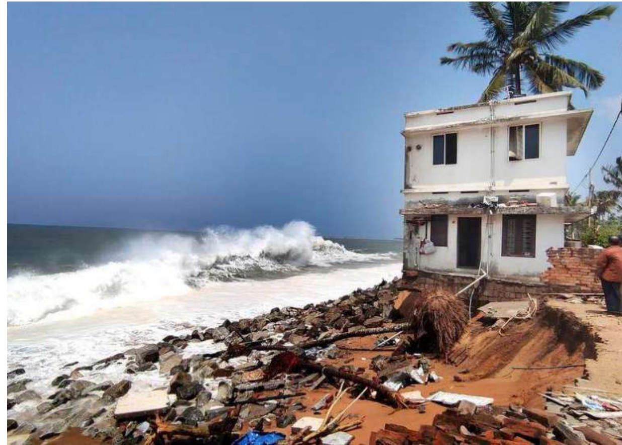
Skeletal structure: Houses destroyed by a sea surge on Monday at Mundakkal in Kollam, Kerala. C. SURESHKUMAR
