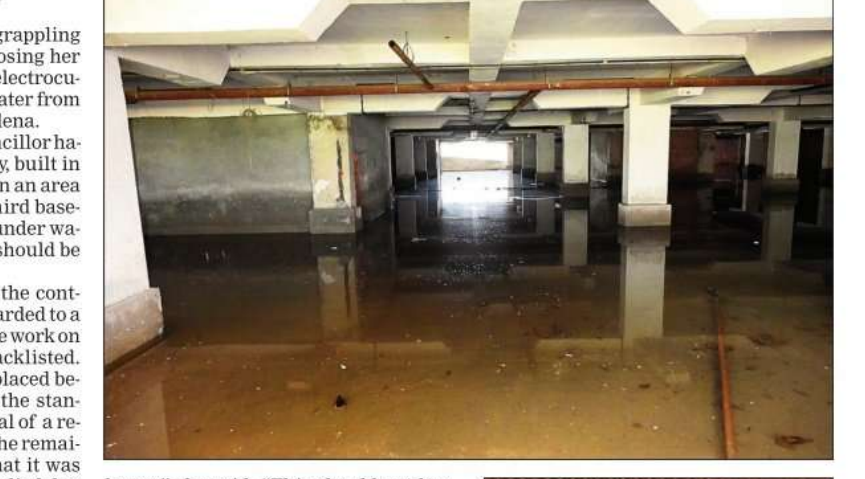
Kartik (25) was electrocuted while trying to pump out water from the parking lot
