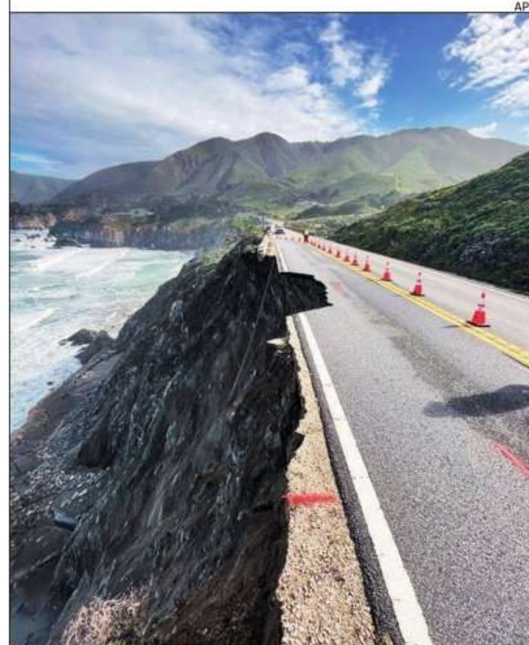
A portion of scenic Highway 1 in the Big Sur area of California collapsed Saturday, stranding about 2,000 motorists, mostly tourists, overnight. The highway, also known as the Pacific Coast Highway, features stretches of rocky cliffs, lush mountains, panoramic beaches and coastal redwood forests. Large chunks of the road fell into the ocean. Officials did not say what led to the collapse, but torrential rain had battered the area. There were no reported injuries. On Sunday, uniformed officials were guiding some motorists around the damaged road in organised convoys. NYT
